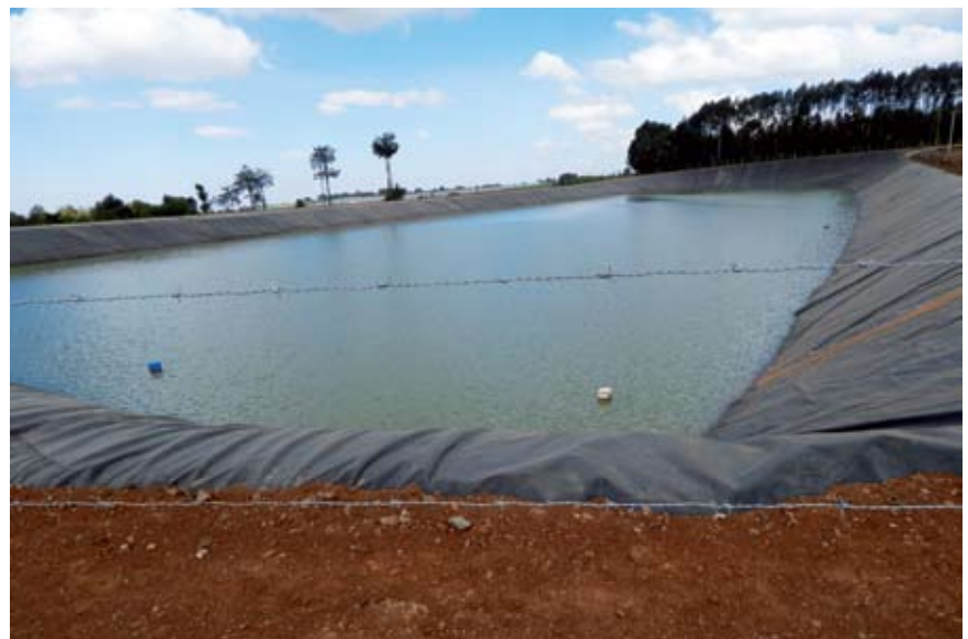
Reservoir with an impressive capacity: This consists of rainwater collected from the Greenhouses.
