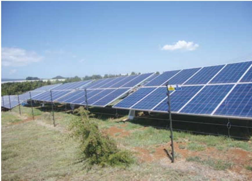
Solar Panels at Timaflo Ltd
